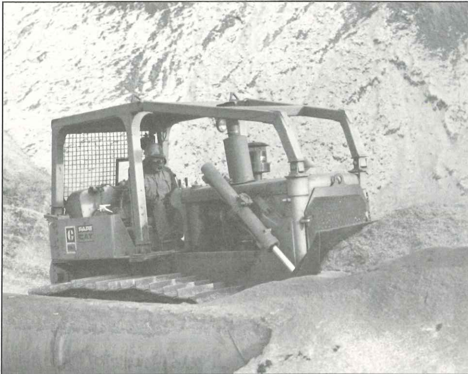
Dan Dickman pushes hog fuel onto conveyor at the powerhouse.
