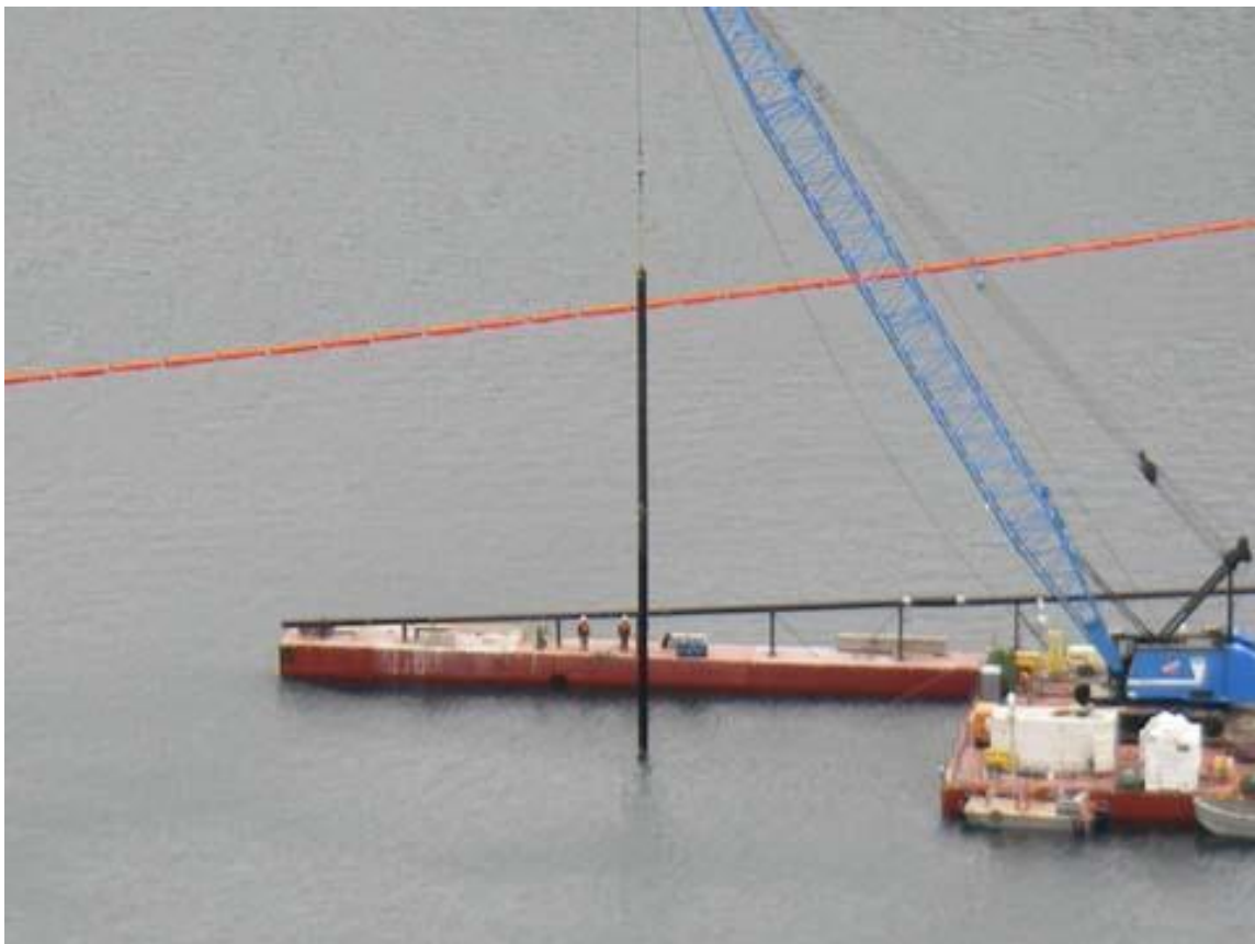
A crane barge excavating 250 feet below the surface of Lake Billy Chinook at the Round Butte Powerhouse intake structure.
