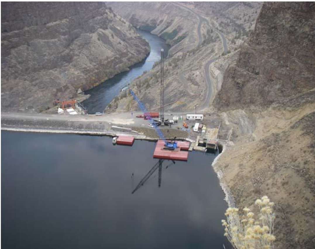
Crane barge used to erect the temporary platform for the construction of the intake structure on the selective water withdrawal tower.
