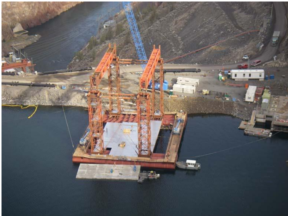
Temporary barge platform used to construct the bottom structure. It will also be used to construct the vertical flow conduit.
